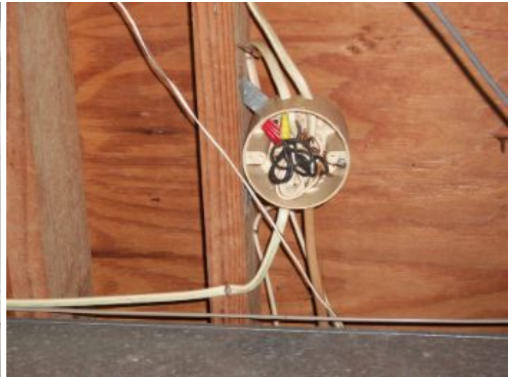
Junction box missing cover plate in garage.
