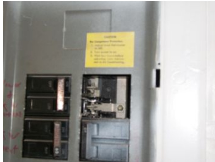
Missing Breaker knock out.
