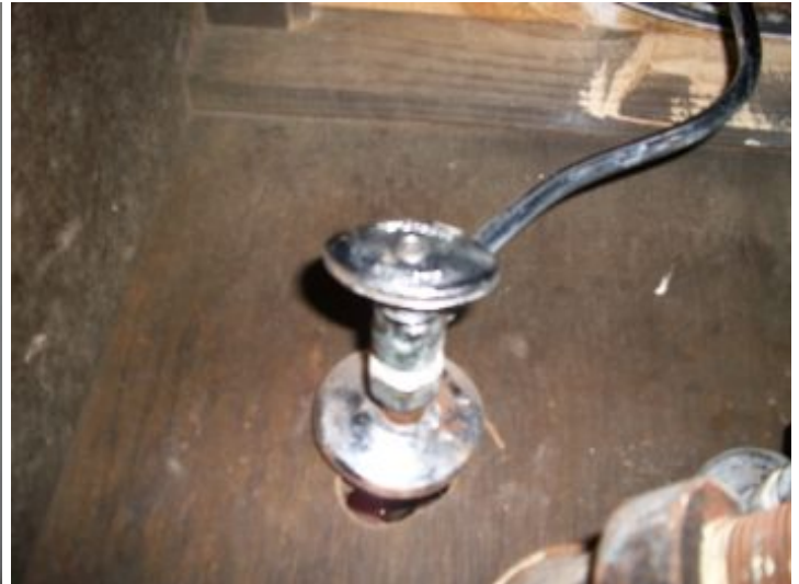
Supply line leak under the downstairs bathroom sink.
