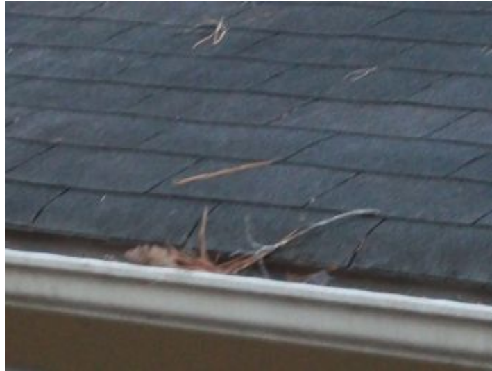
Gutters full of debris.
