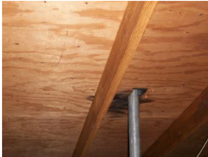
Moisture stain around the vent pipe in the attic.
