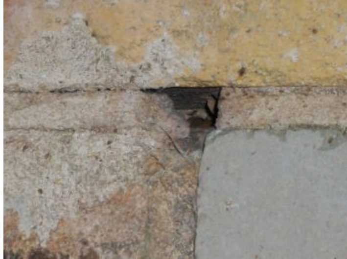
Areas of the brick veneer needs pointing.
