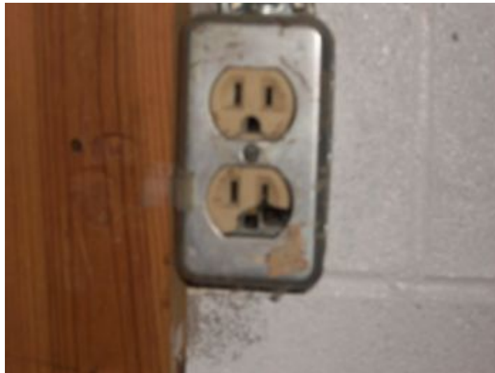
Outlet damaged in garage.
