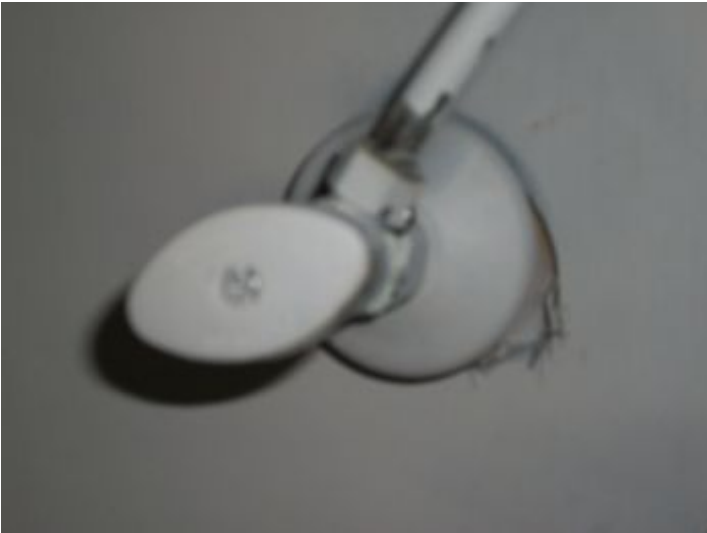
Supply line under hall bathroom sink leaking.
