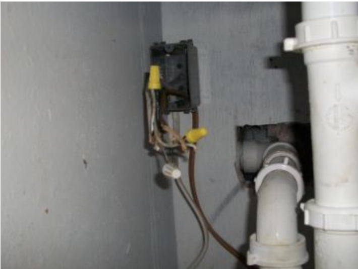
Junction box missing cover plate under kitchen sink.
